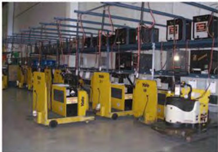
■ The electrical battery charging room.
