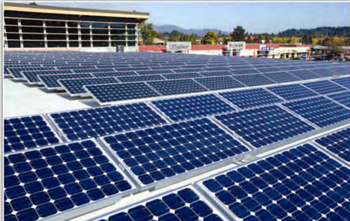
■ SOLAR PANELS - Since 2009, Market of Choice has been using 562 rooftop mounted SolarWorld 175-watt photovoltaic solar modules to generate electricity.
