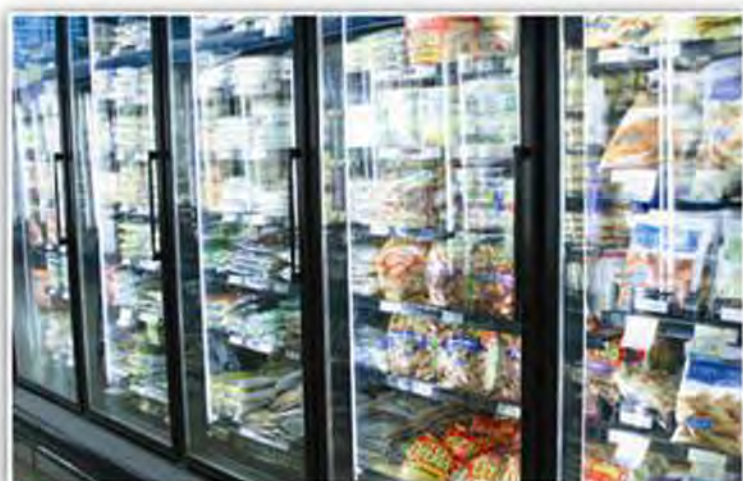
■ FREEZER DOOR NEW LIGHTS - Market of Choice typically uses energy-efficient refrigerated cases by Hill Phoenix, Conyers, GA, with fluorescent lighting.
