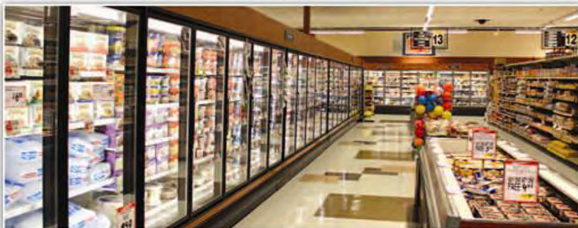
■ New LED coolers will help the store save 30 percent on energy costs.
