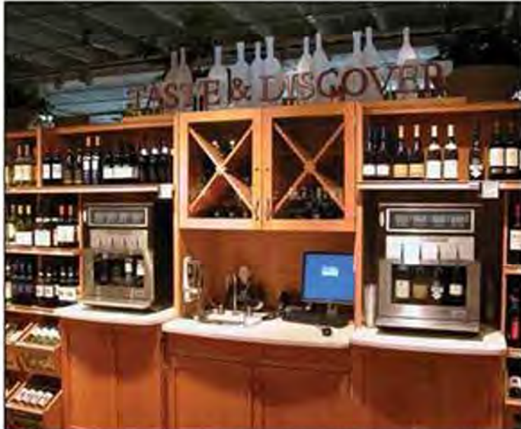
■ A typical wine station installation by Napa Technology. Napa Technology recently released key findings from its recent retail survey during a thought-provoking webinar centered on wine consumption trends.
