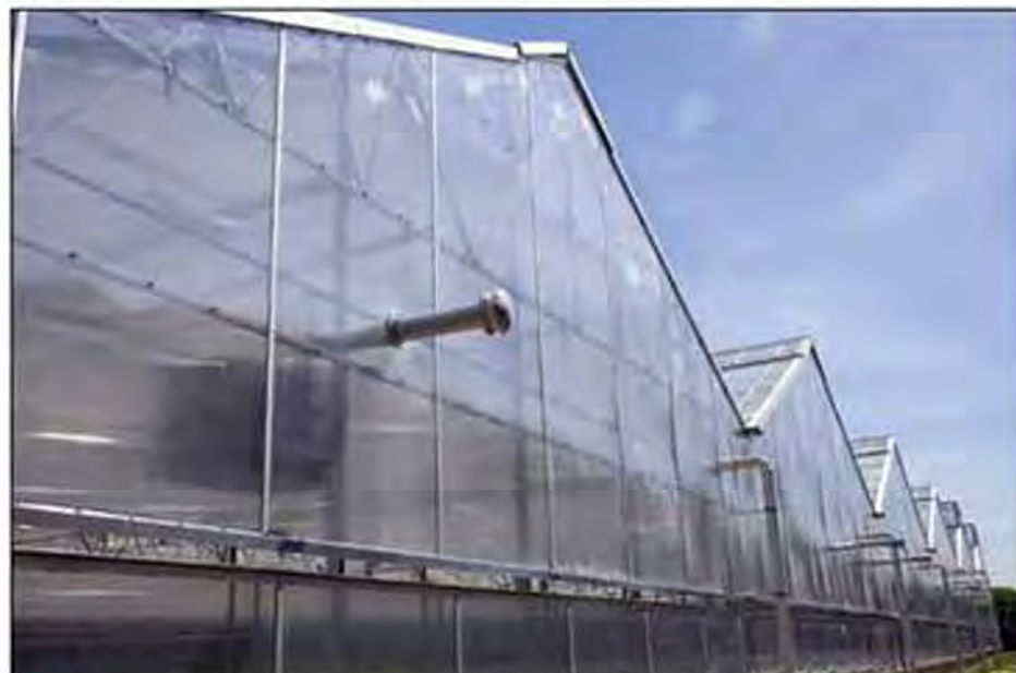
BRIGHTFARMS, INC is upgrading its greenhouse in Bucks County, PA. With this upgrade, BrightFarms is installing state-of-the-art growing systems and harvesting equipment. The objective of this upgrade is to more efficiently grow baby greens of superior quality.
