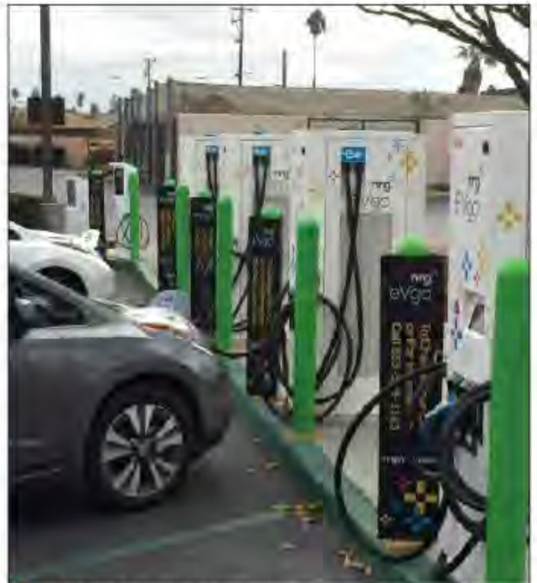
QUICK CHARGE - Located in the hottest electric vehicle (EV) adoption area of the country, the Lucky Fremont location at 5000 Mowry Ave. features four 50kW DC Fast Chargers able to charge vehicles at the same time.
